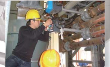
Steam system for boiler use
