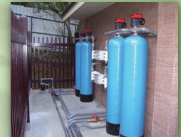
Water treatment system
