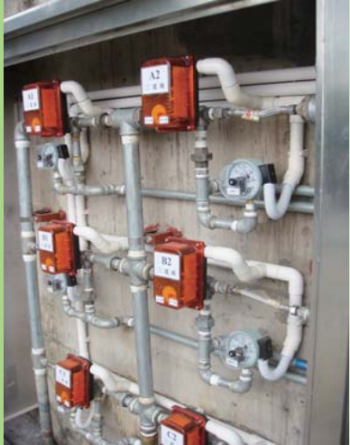
Filter system for waterworks in Guangzhou
