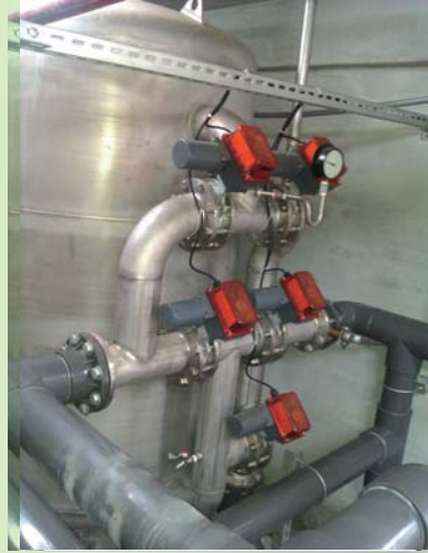
Filter system in National university in Taiwan
